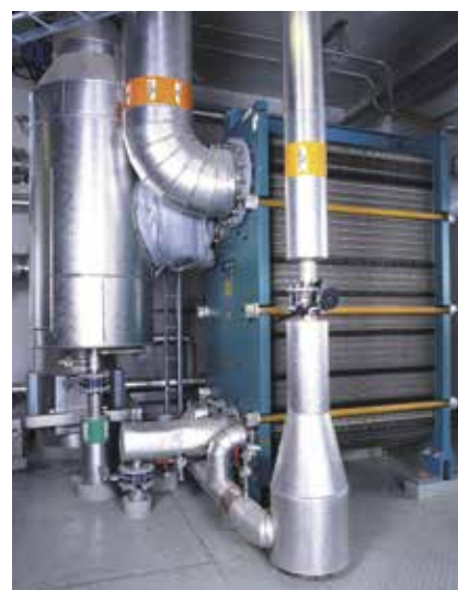
Ethanol condenser at The Absolut Company in Sweden. All the columns at The Absolut Company's Åhus distillery use Alfa Laval reboilers and condensers. The Alfa Laval units were chosen because of their compactness compared to corresponding shell-and-tube solutions.
