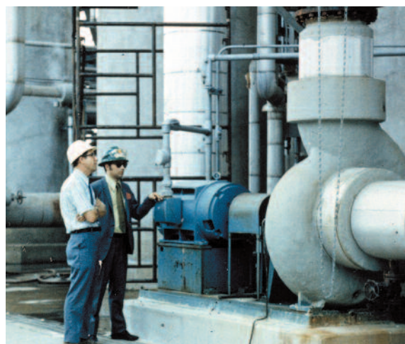
A 3175 installed in a major chemical plant.
