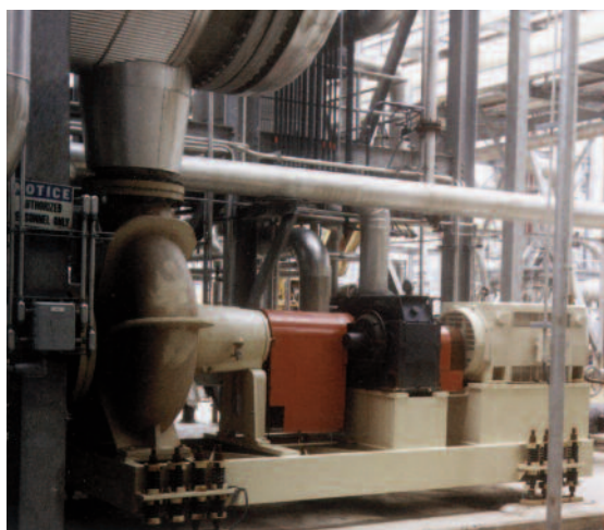
Black liquor circulation pump (3175 XL) on spring-loaded baseplate.
