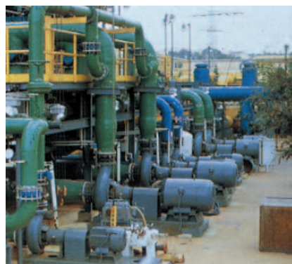
3175's on process service such as multi-effect evaporators.
