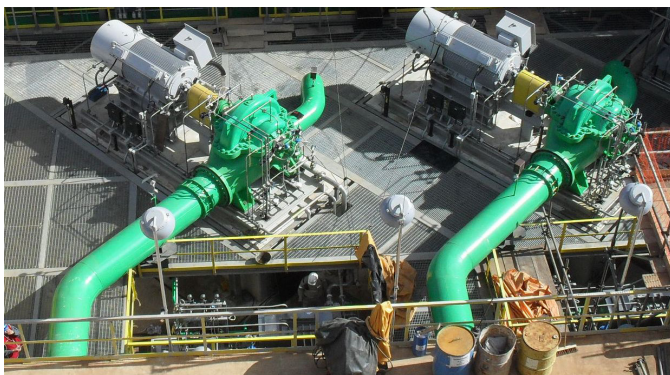
Brazil Refinery Cooling Tower Service
