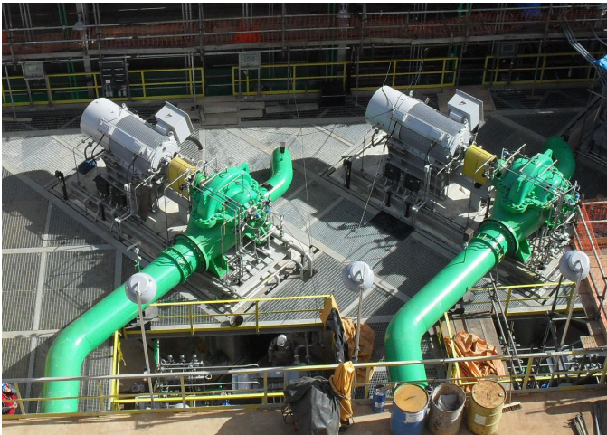
Refinery Cooling Tower Service (Brazil)
