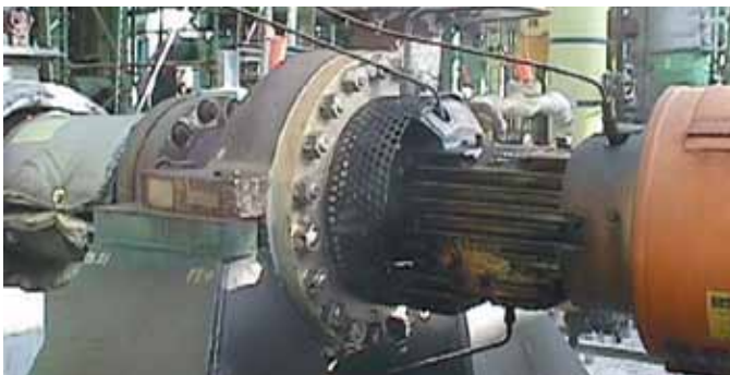
Model 3700 on high-temperature service at a U.S. Gulf Coast refinery.
