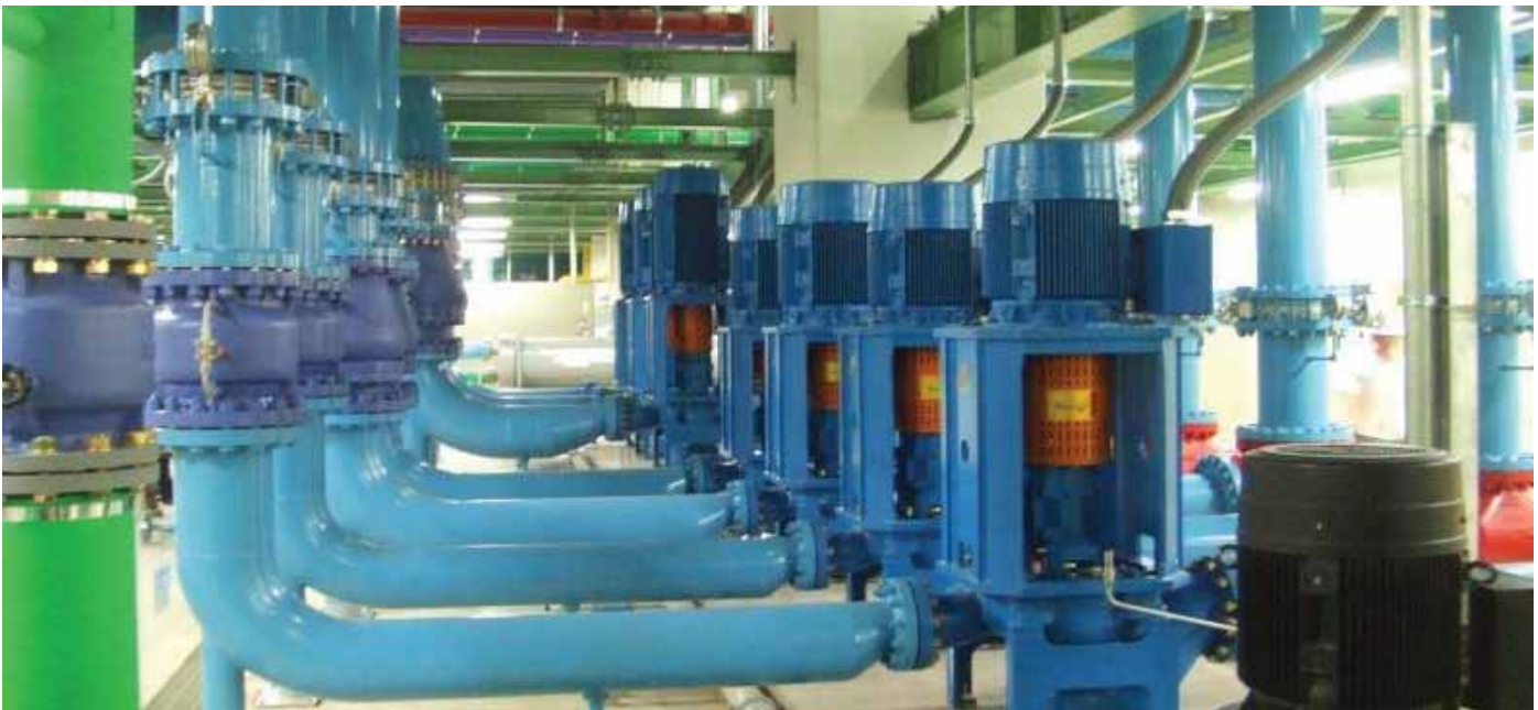
This ITT Goulds customer saved space as well as foundation and baseplates costs with seven Model 3910s. Many applications benefit from the inline piping as well.
