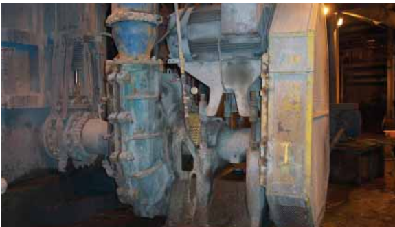
SRL-XT 14×12–36 on Ball Mill Discharge Service
