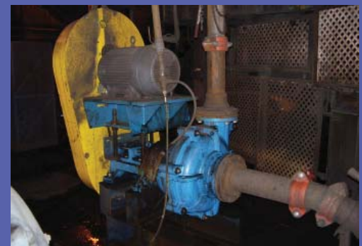
Thickener Underflow Pump in a Coal Preparation Plant
