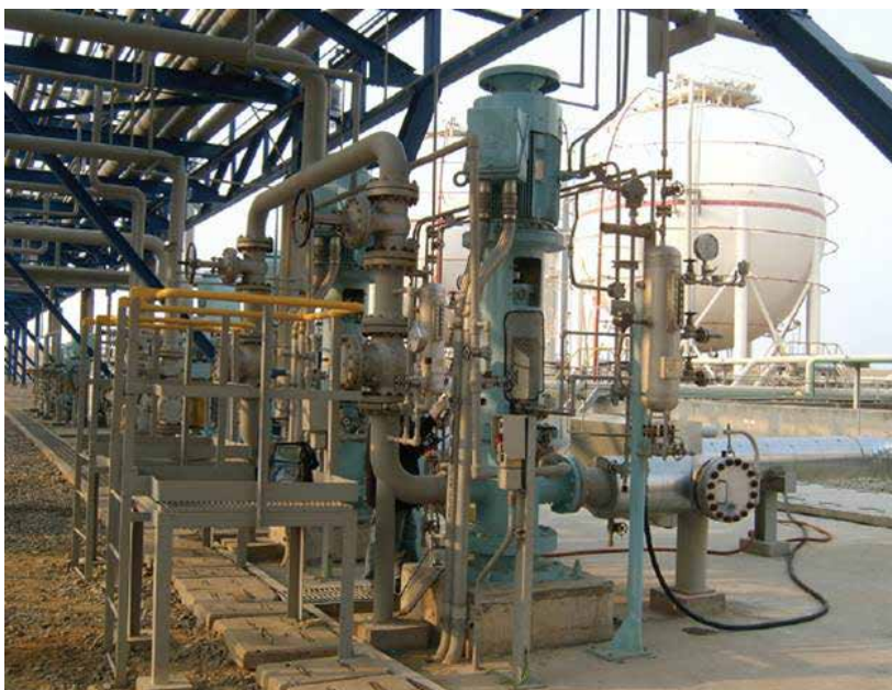
Many of these high head applications involve pumping low specific gravity hydrocarbons in a VS6 suction can arrangement.
